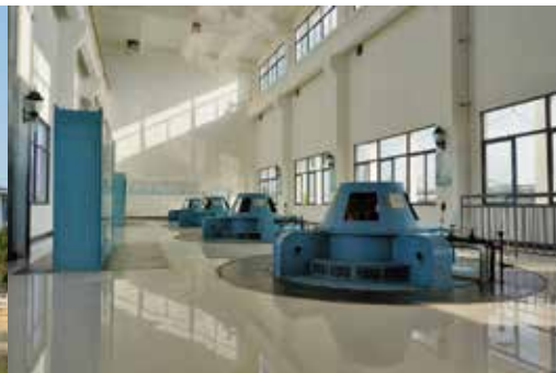
Wuhu Longwo Lake Pump Station
