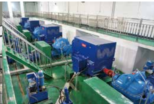
Beijing Xingshikou Pump Station
