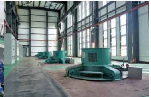
Tianjin Beitang Pump Station
