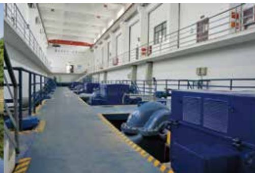
Zhengzhou Zhongyuan West Road Pump Station of The South-North Water Transfer Project
