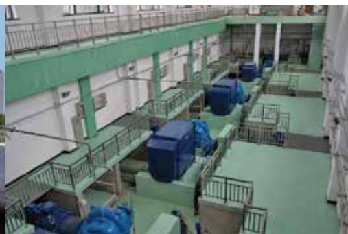
Beijing Yuquan Mountain Pump Station of the East-West Water Transfer Project
